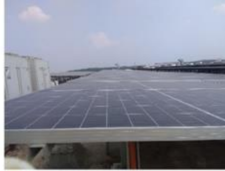
Roof top solar supplier site, Pune
