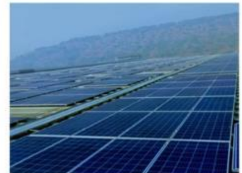
Roof top solar @ supplier site, Pune
